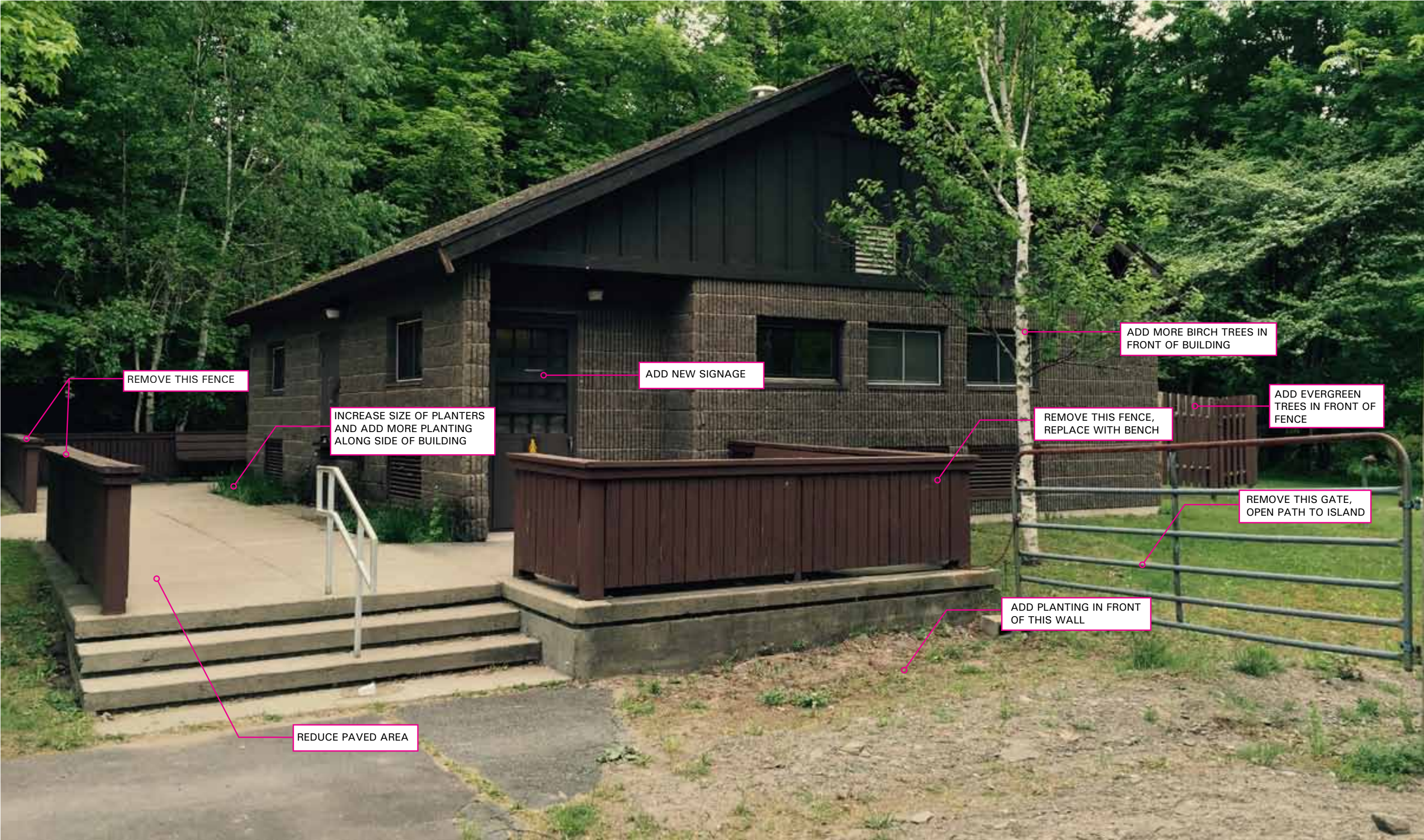
WASHROOM BUILDING RECOMMENDATIONS
