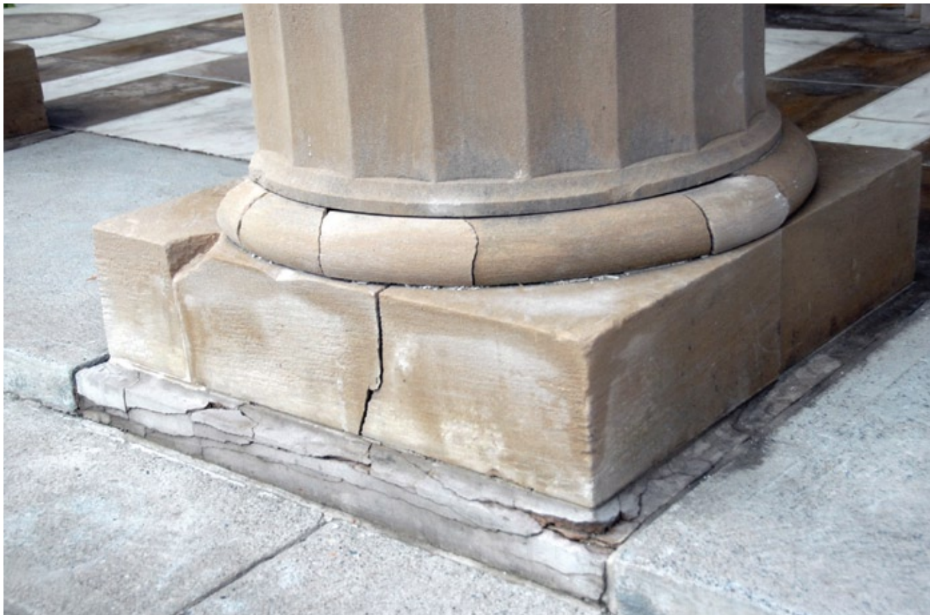
A column in need of repair at Saratoga Spa State Park
